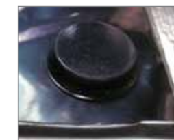
Placed 3M Bump-on Stoppers at corner edges of the frame to prevent direct contact to wall surface allowing air circulation
